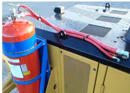
Figure 15 Externally mounted hosing and spiral wrap.
