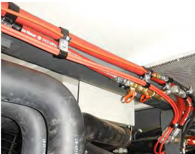
Figure 14 Internally mounted hosing.
