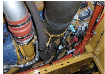
Figure 16 Hosing protected with fire sleeve.
