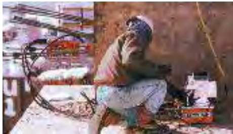
The PE60 used for pre-stressing.
